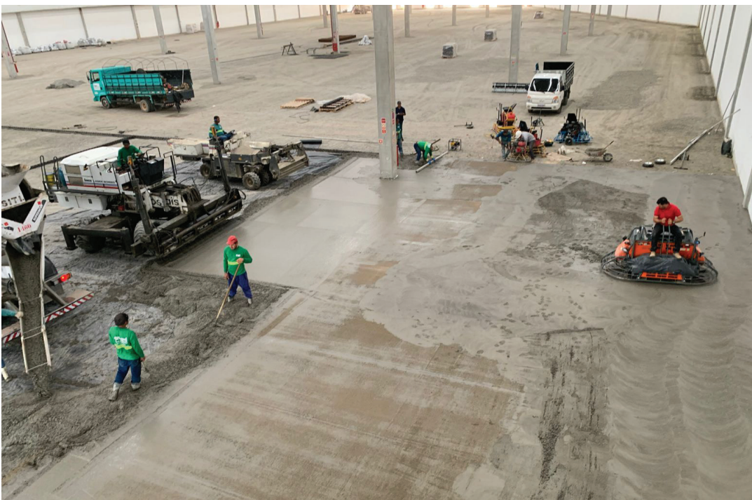
A ride-on power floating machine with hardener, shake-on machine, laser screeder and concrete being delivered.
